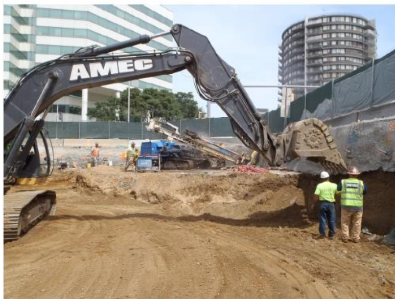
Figure 5: Photo. Digging of a soil raise for the purpose of building a soil nail wall. Images provided by Moretrench American Corporation [15].
